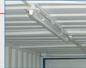
fluorescent light with damp room switch
